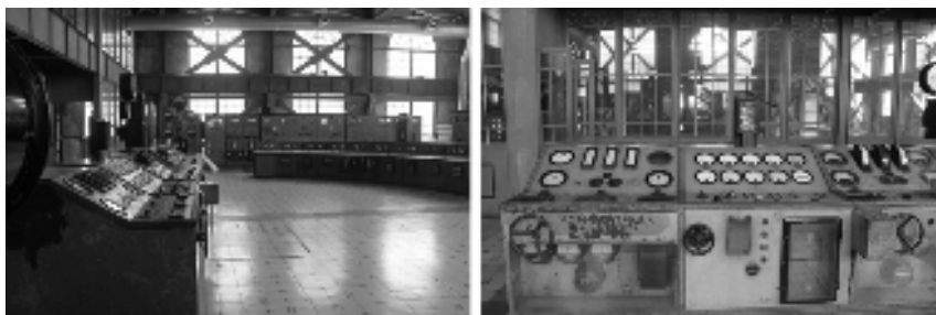
Figure 7: Interior of the control room
