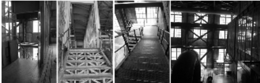
Figure 3: Stairs to machine hall
